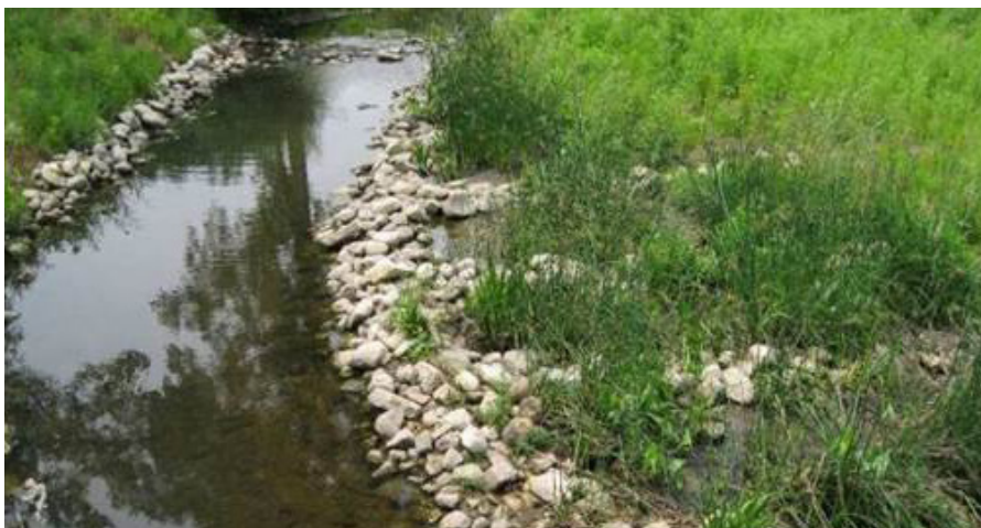
“Rock toe” stabilization around a lake edge
